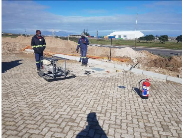
Image 14: Generator in use with a drip tray and fire extinguisher
