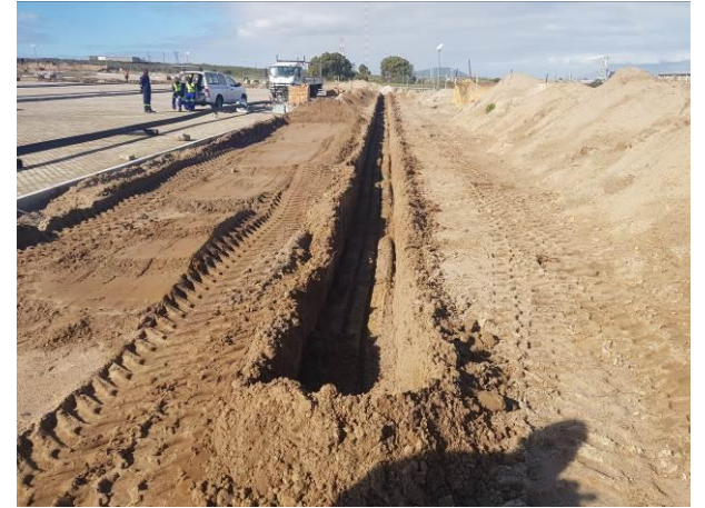
Image 9: Undemarcated trench on site
